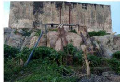
Shiroro Tank showing outlet pipelines for DMA bulk meters
