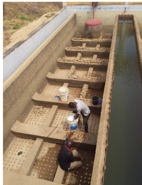
Exhibit 39. Imo SWC completing rehabilitation of Owerri's Otamiri WTP filtration process through the USF, leading to water production for the first time in 7 years.
