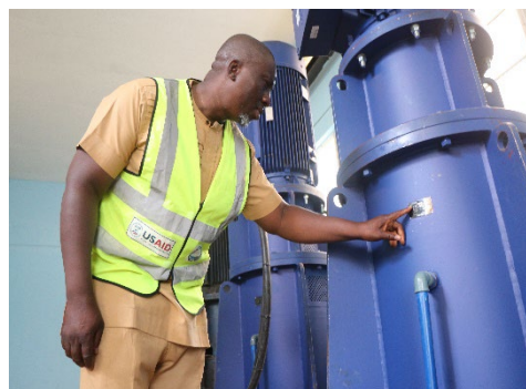
Exhibit 12. ISWSC monitors new pumps as part of its asset maintenance management program.
