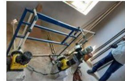
Installed HTH Dosing pumps
