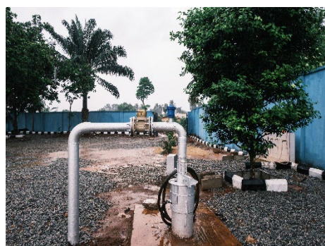
Exhibit 85. This new borehole constructed in Issele-Uku in Delta was funded by the USF and is already tracked in DESUWACO's asset monitoring database in its ERP system.
