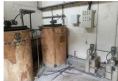
Rehabilitated Chemical Dosing Unit
