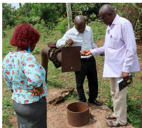
Exhibit 30. Assessments of water production and distribution schemes, such as this unused pipe in Delta, informed the preparation of priority technical and infrastructure support activities.
