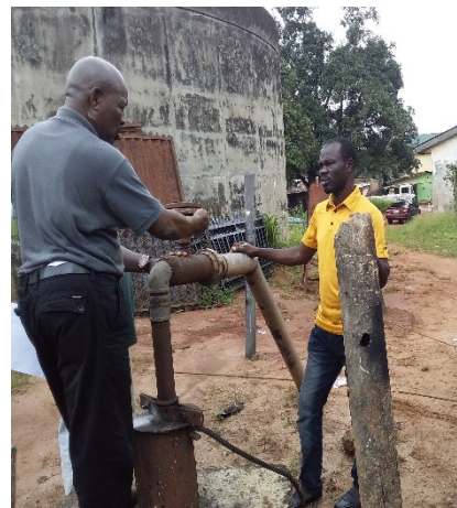
Exhibit 77. DESUWACO staff reviewing its assets as part of technical assessment for performance monitoring.
