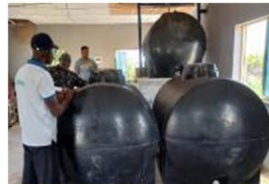
HTH mixing tank with stirrer & dissolution tanks
