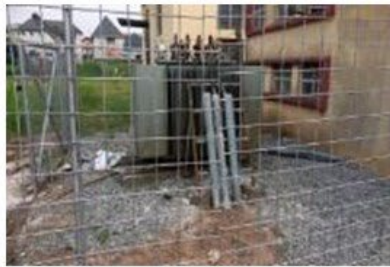
Rehabilitated 1,600 KVA Transformer
