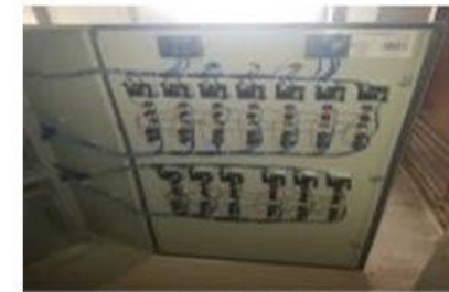
Control Panels at Bi-water & Impressit WTPs
