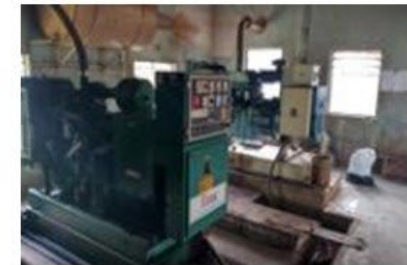
Rehabilitated 160KVA & 200 KVA Gen-sets
