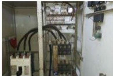
Transformer and Generator Change over Panel
