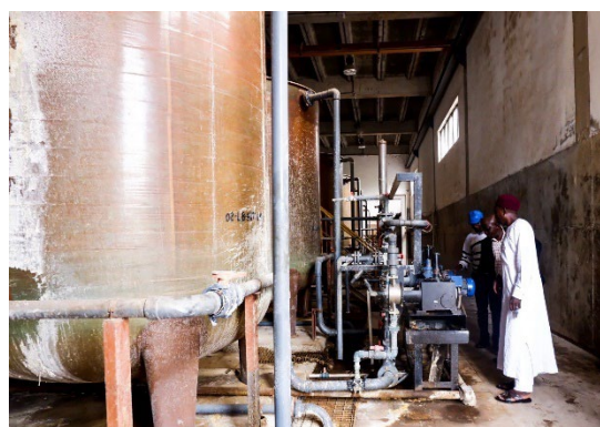
Exhibit 37. Critical technical and institutional assessments of water schemes by specialized experts provided evidence for co-design of technical and infrastructure support.
