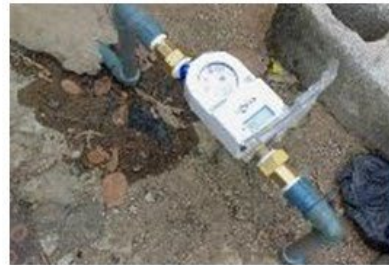
Installed prepaid meter
