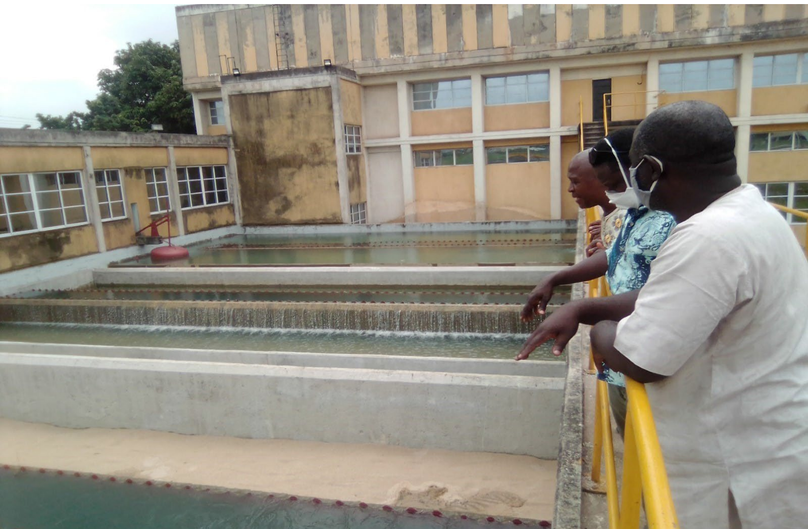
Filtration system at Otamiri Water Scheme/Treatment Plant, Owerri, Imo State (Photo credit: Engr. Tony Offor; August 18, 2020).
