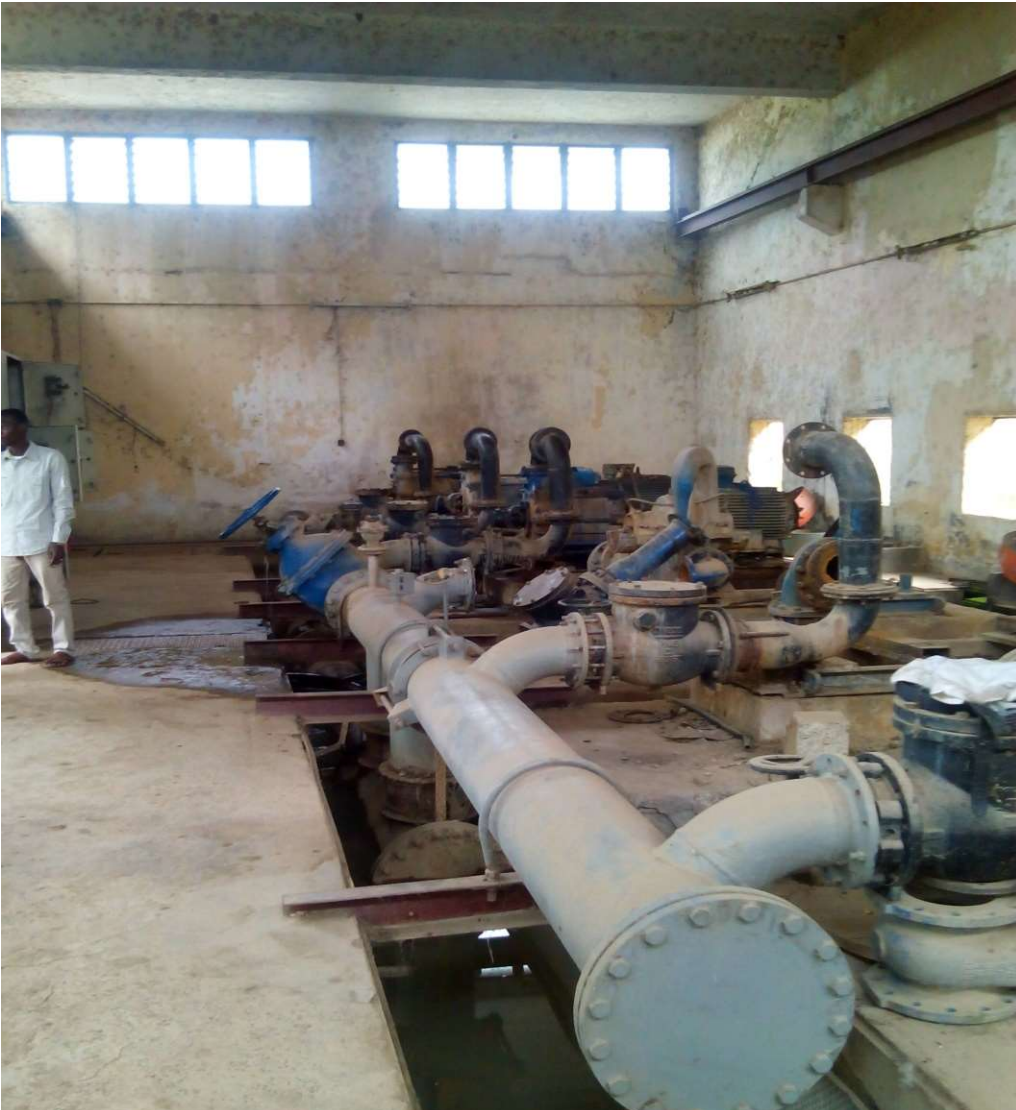
Yola Treatment Plant (6 high lift pumps with only 2 working)
